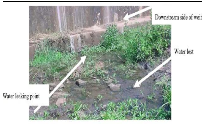
Fig. 4. Leakage on river diversion structure
