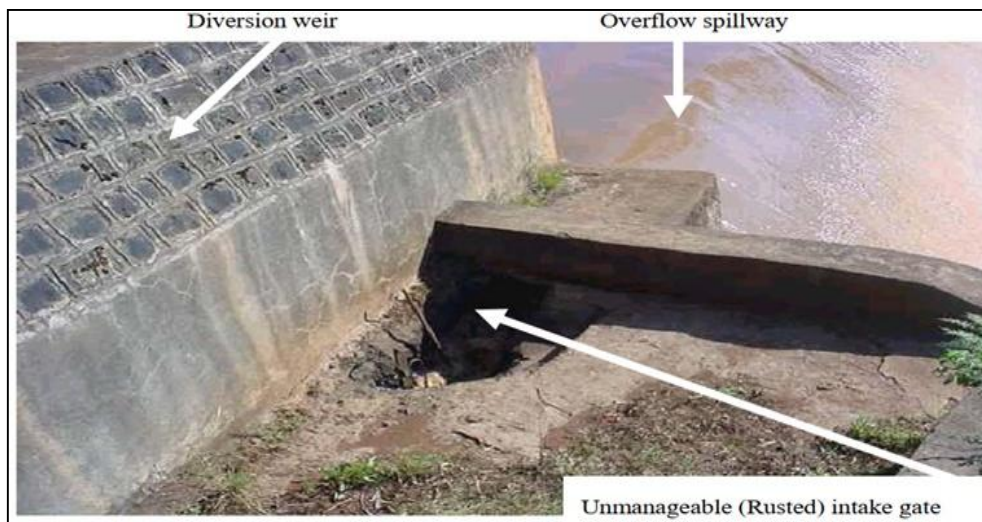
Fig. 1. An intake gate of diversion head work
